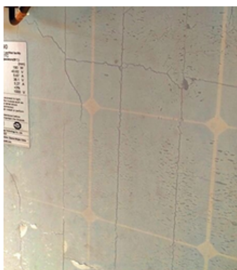
Figure 01 : Back sheet cracked solar panel
